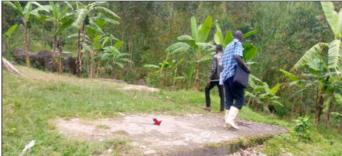
Fig. 2. Representative images of the remains of Nametsi Health Center II (Red Arrow), that was sunk by landslides in Bududa District, Eastern Uganda
