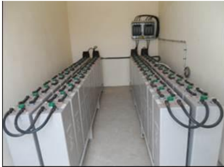
Fig. 3. The two battery chains
